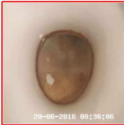
5.1.1 Scrapes To Upper Wall LHS Of Window.
